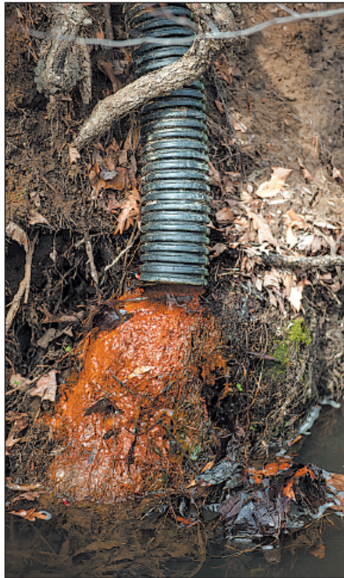
By Matthew Cole, Staff A section of drain tile deposits stormwater into Beaver Creek from Crofton Country Club.
